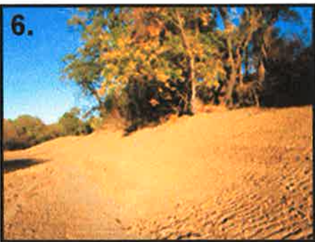
6. The out-of-place channel after fill and slope applied toward Putah Creek Road. Seeding was completed after this image was recorded.
