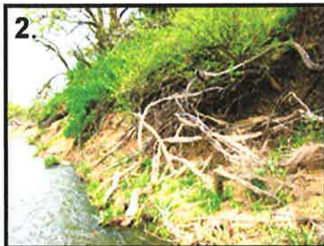
2. Closeup of the section of Putah Creek that was undermining Putah Creek Road.
