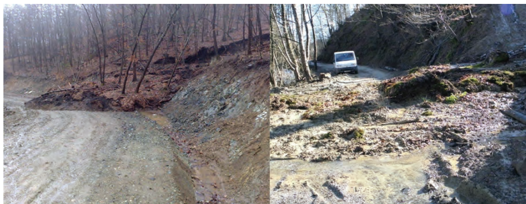
FIGURE 4. Left: Damages on forest road caused by landslide. Right: Damages on forest skid-trail
