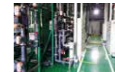
Initiative by Dalian Seiko Instruments Inc.: Investment in state-of-the-art factory wastewater treatment facility
