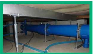
Drinking water storage system
