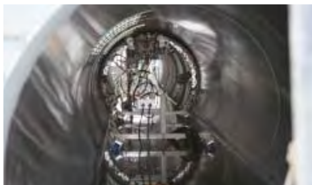
The pipeline renewal business is expanding its offerings of new construction techniques and products (Photo: The automated SPR method).
