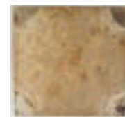
SUS304 Small amount of red rust (No effect to the function)
