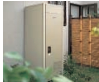
Electric Hot Water Unit
