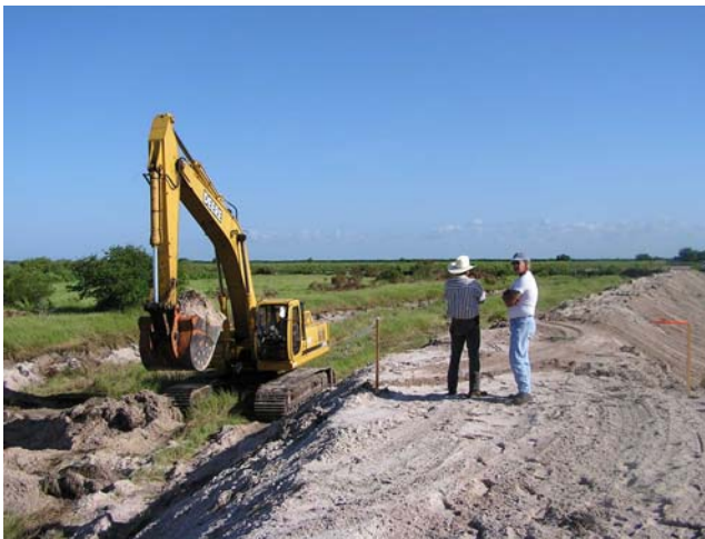
The picture above depicts construction of the perimeter berm around D1 and D2 from the ground.
