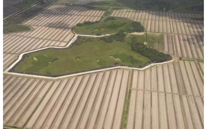
The picture above is an aerial overview of the J-7 Ranch Project's D-1 and D-2 retention area during construction. The white line around the green area is the retention area's perimeter berm.
