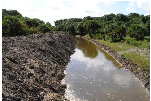
The picture above depicts a portion of the Toney Strand Project after sediment removal and cleaning.
