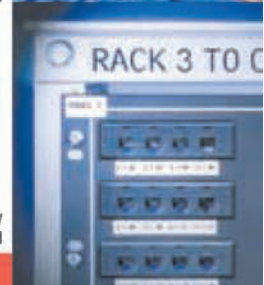
Racks clearly identified
