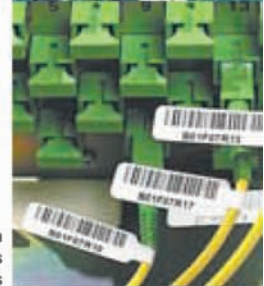
Data communications equipment labels
