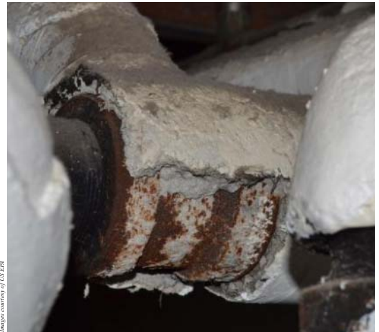
Top from left: Warning on a building, contaminated with asbestos; Asbestos fibres may be released into the air by the disturbance of asbestos-containing material during product use, demolition work, building or home maintenance, repair, and remodeling; Asbestos pipe wrap (joint partially removed).
