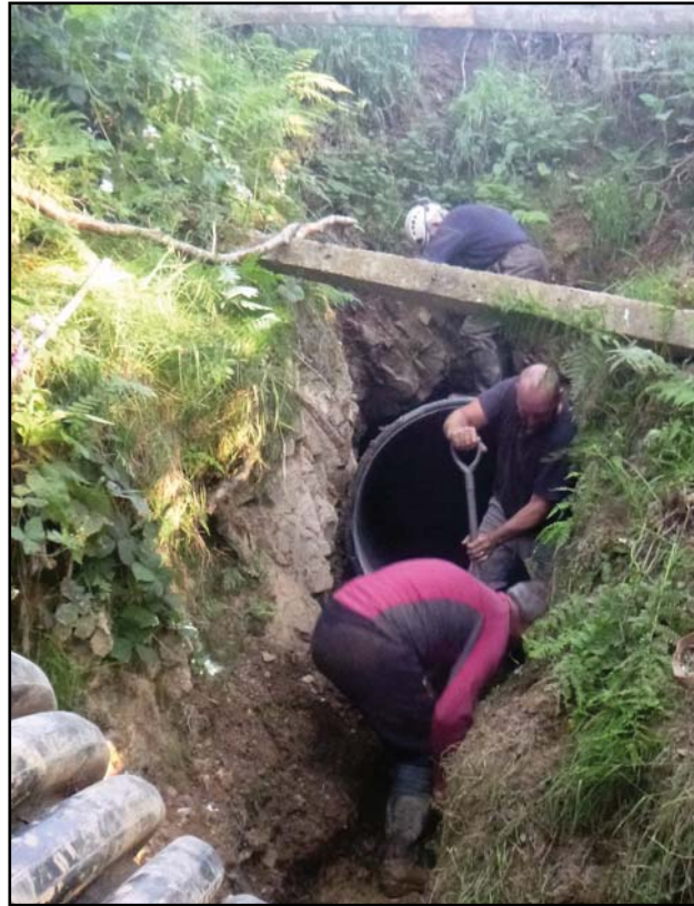
Left: Digging in the entrance to Yew Tree level on the 4th July. (Nick Southwick)
