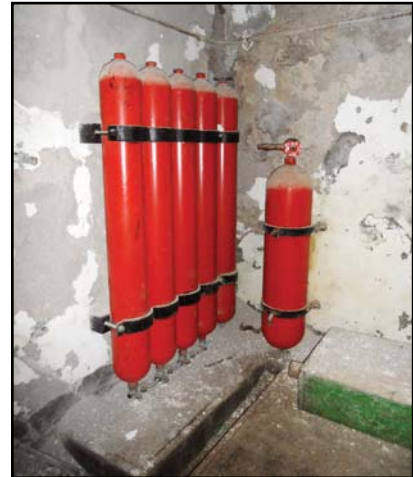
Above: Gas cylinders in the generator room.
