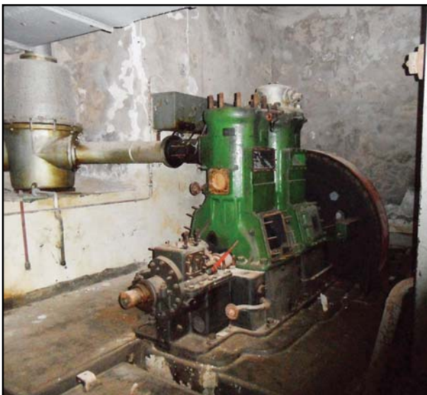
Above: The 25hp diesel engine driving a dynamo to produce 110 volts DC for the hydraulic power and lighting.
