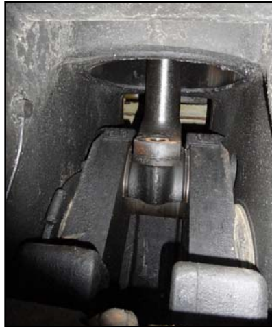
Above: Crank of the 25hp diesel generator.
