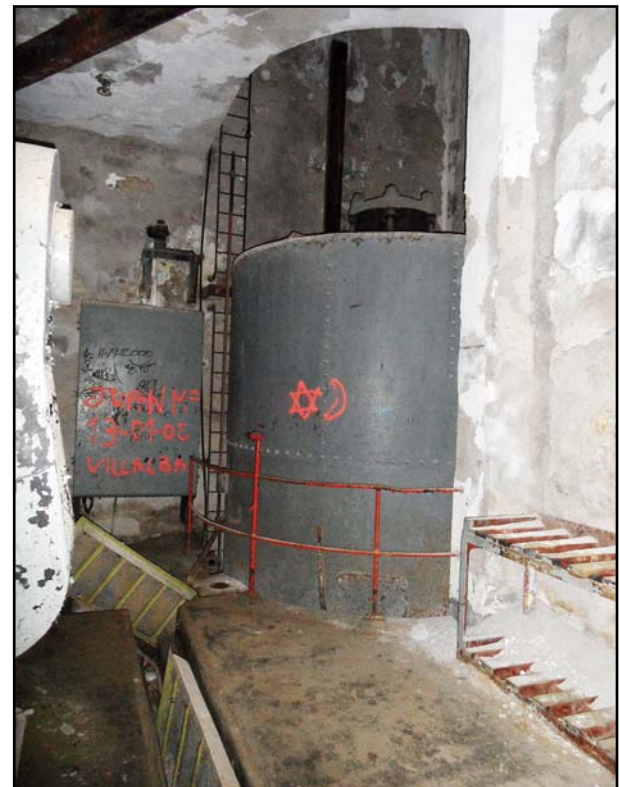
Right: Diesel tank and the hydraulic accumulator/reservoir?
