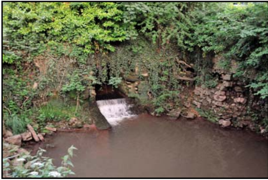
Figure 4: Drainage culverts in the wall of the basin, with Paper Mill brook emerging from its culvert. (Kelvin Lake - I.A.Recordings)
