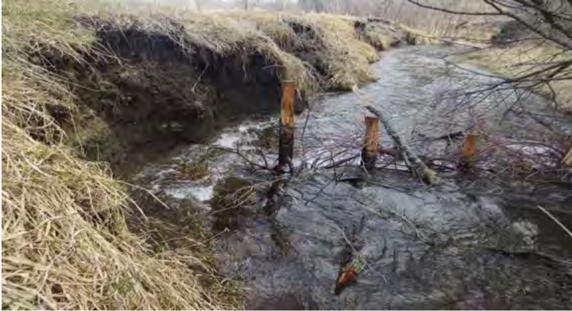
Figure 78: Breach of BDA 1 showing water flowing around the structure, eroding the left bank. This BDA is still functioning as grade control through water impoundment upstream as well as facilitating the widening of the incision trench. Notice the development of an inset flood plain directly downstream along the right bank
