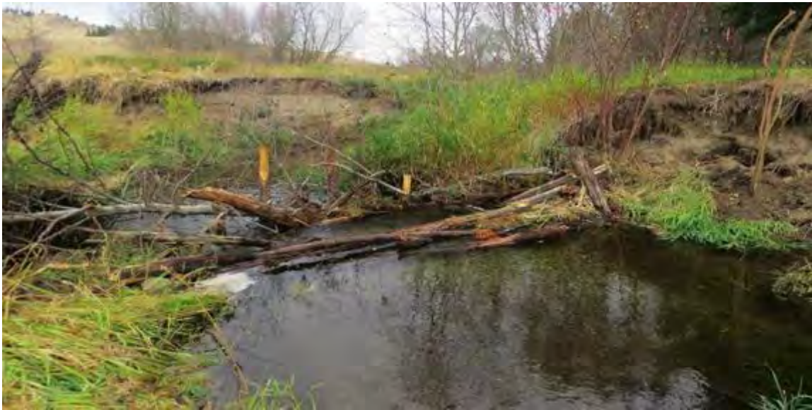
Figure 77: 12 days following installation of a BDA (same location as figure 81) and placement of LWD and other debris showing water pooling upstream
