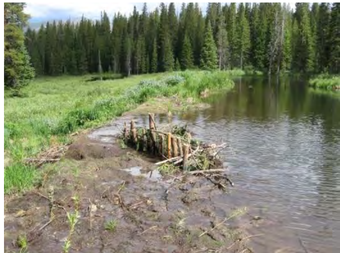
Figure 63: A PLWW was constructed on one repaired dam to temporarily fortify a nick point while we were waiting for beaver to reoccupy the site
