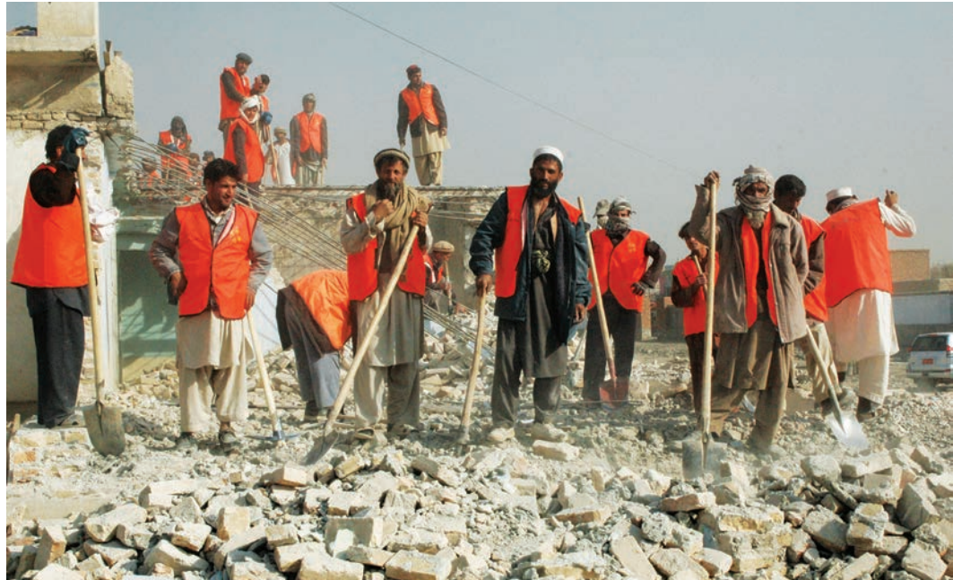
Afghan construction workers help build the Kabul National Cricket Stadium. (USAID photo)
