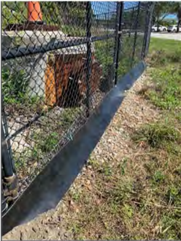
Figure 9. Conveyor Belt Installed at Side Gate
