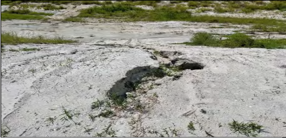
Figure 1. Berm Rill Created from a High Rainfall Runoff Event
