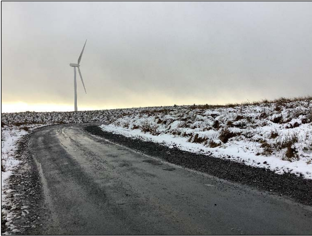
Plate 13-77 Continuation of proposed construction access road along existing road where upgrade works are required, looking south
