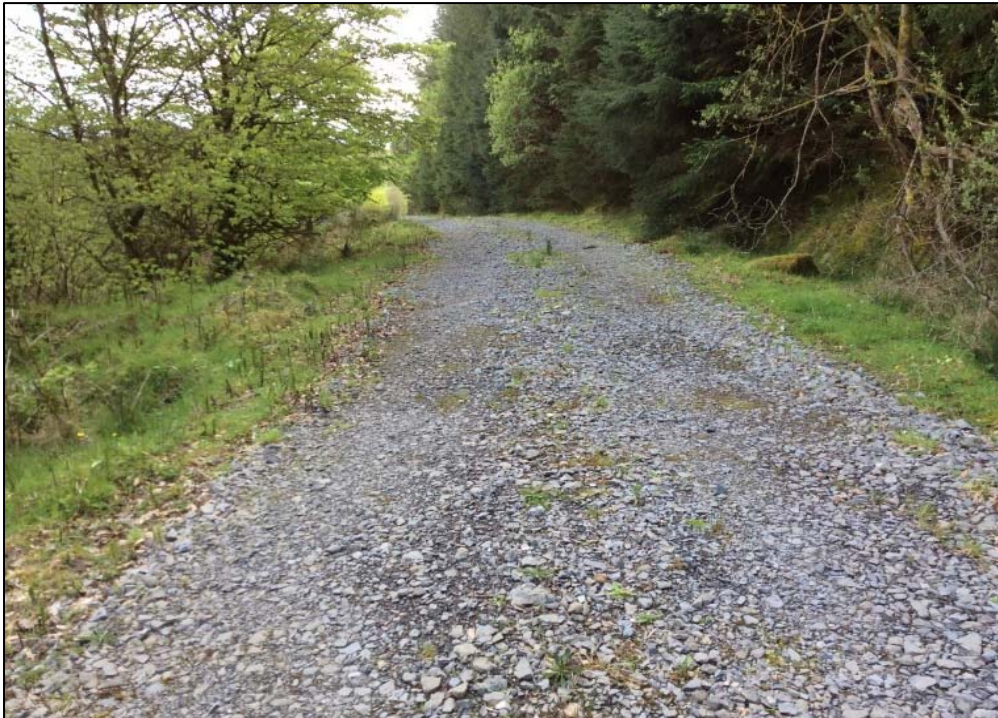
Plate 13-65 Continuation of construction access road looking SE along existing section of road.
