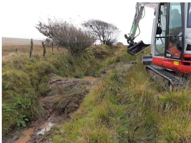
Excavator blocking a ditch on Exmoor ©Conrad Barrowclough
