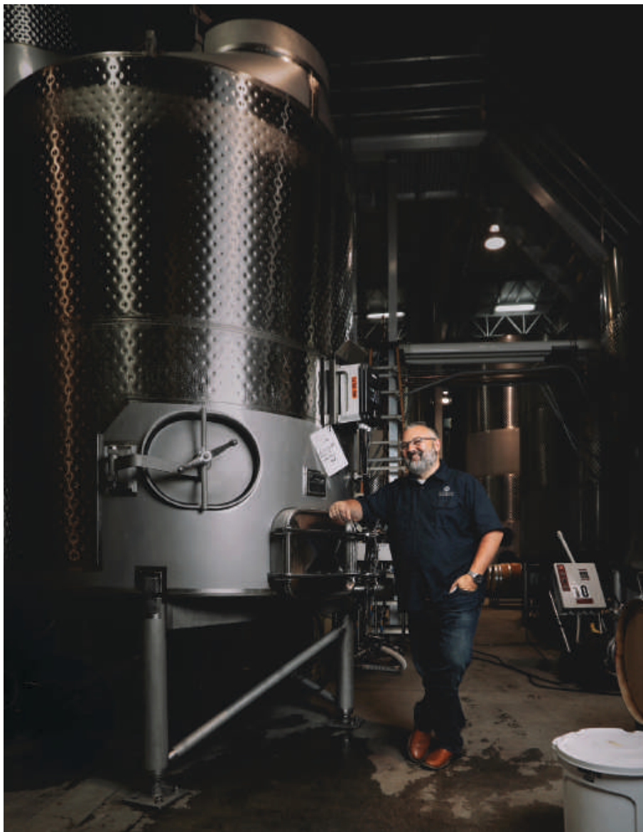
All tanks aren't created equal: With features like dimpled jackets, dual screens, TankNET controllers, and dedicated pumps, these custom-built 7-ton fermenters are well equipped to handle Herzog's luxury tiers.
