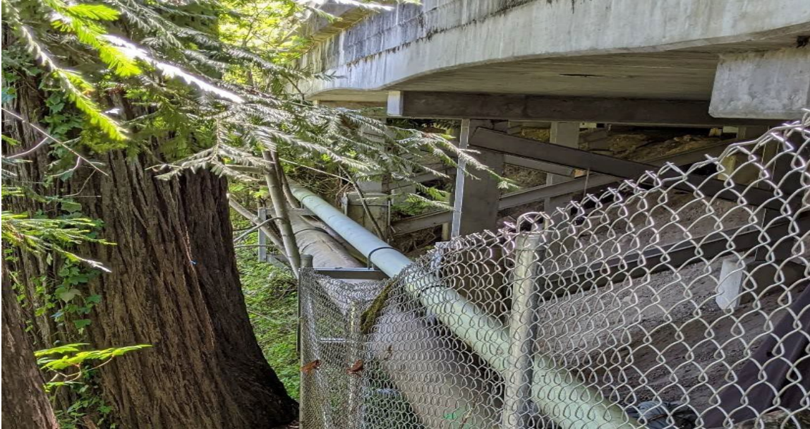
Figure 14. The existing 16-inch diameter steel Main Force Main and 8-inch diameter gravity sanitary sewer suspended along the Hwy 116 viaduct.
