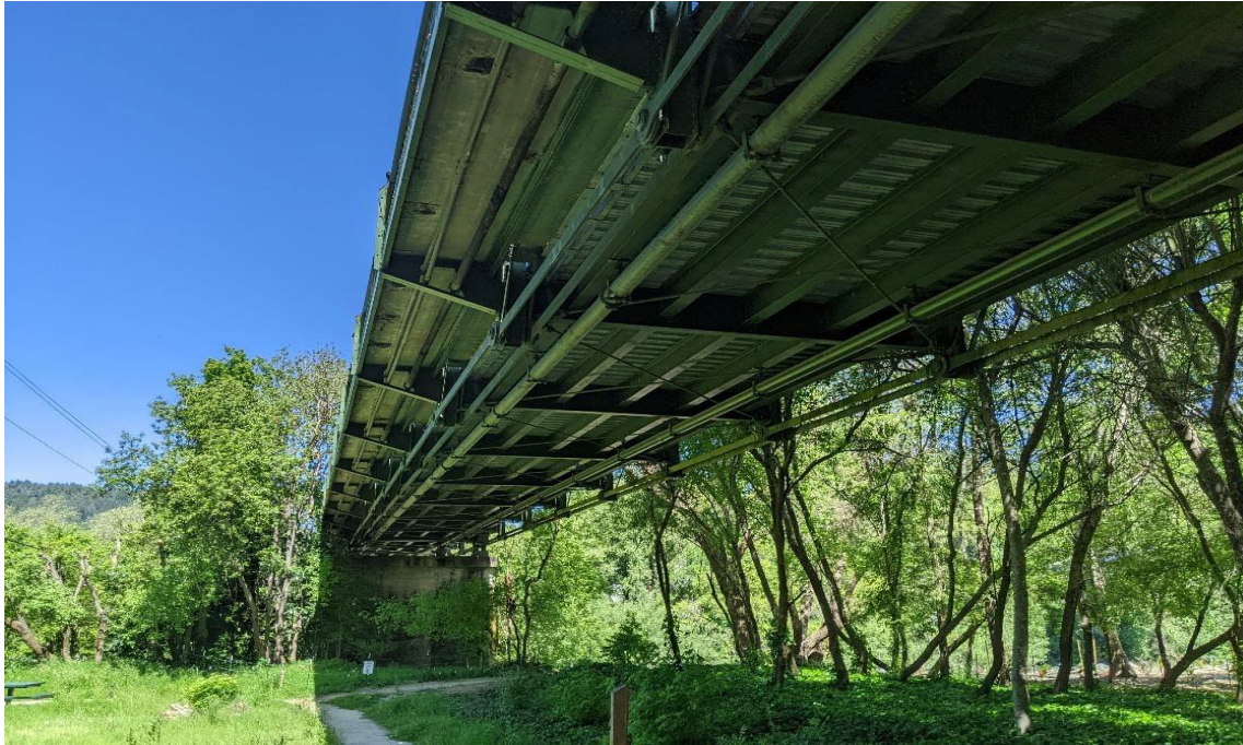
Figure 9. Looking northwest under the Guerneville Bridge at the existing Beanwood Force Main hanging on the underside.
