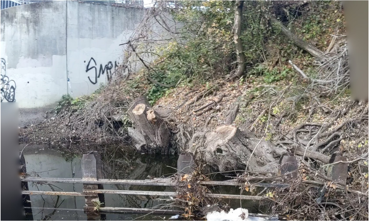
Photograph 2.2-6. Scour at Right Bank (Looking Downstream) at E Street Bridge Fishway Extension.
