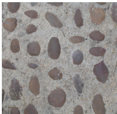
Incorrect river pebble paving
