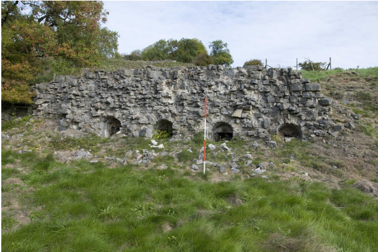
Plate 2: Four of the openings through the downslope retaining wall of the bank of 'ore bins'.
