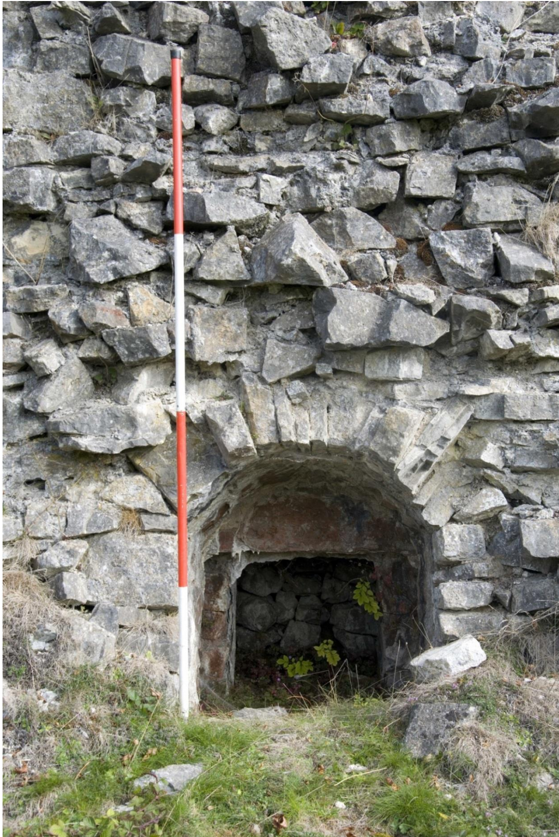
Plate 13: One of the openings into the four ‘ore bins’ to the south-eastern end of the bank of six, with the rubble filling the tank behind visible at the back (Feature J).
