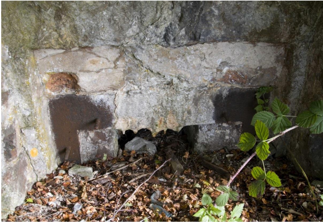
Plate 16: Detail of one of the openings into the two ‘ore bins’ to the north-western end of the bank of six, showing the metal plate and the small inner opening beyond (Feature J).
