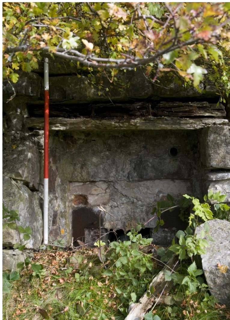
Plate 15: One of the openings into the two 'ore bins' to the north-western end of the bank of six, with an iron plate surrounding the partially choked inner opening visible at the very bottom, with an iron pipe in the back wall above to the top right (Feature J).
