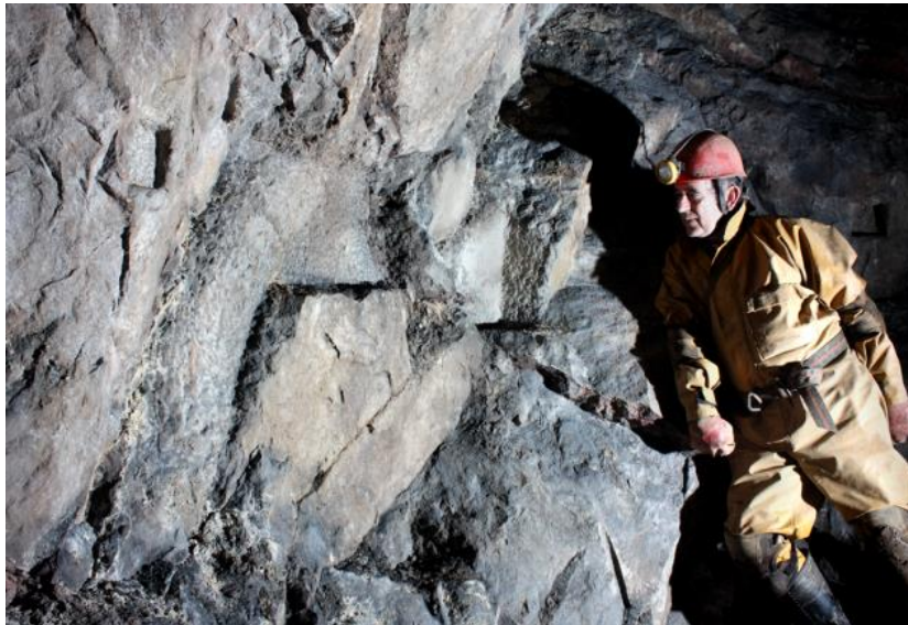
Plate 42: Two of the notches for sturdy paired timbers in the engine shaft chamber, on its north face, which are interpreted as supporting the hydraulic water pressure engine; that to the left has a diagonal slot cut to raise this end of the beam into place. The slot behind at the centre of the photograph had its timber placed from above (Photograph: Mat and Niki Adlam Stiles).
