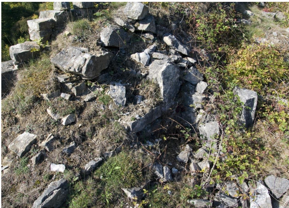
Plate 17: A corner of one of the ‘ore bin’ tanks, with intact walled vertical sides remaining; elsewhere much has collapsed, been robbed or is buried behind rubble (Feature J).
