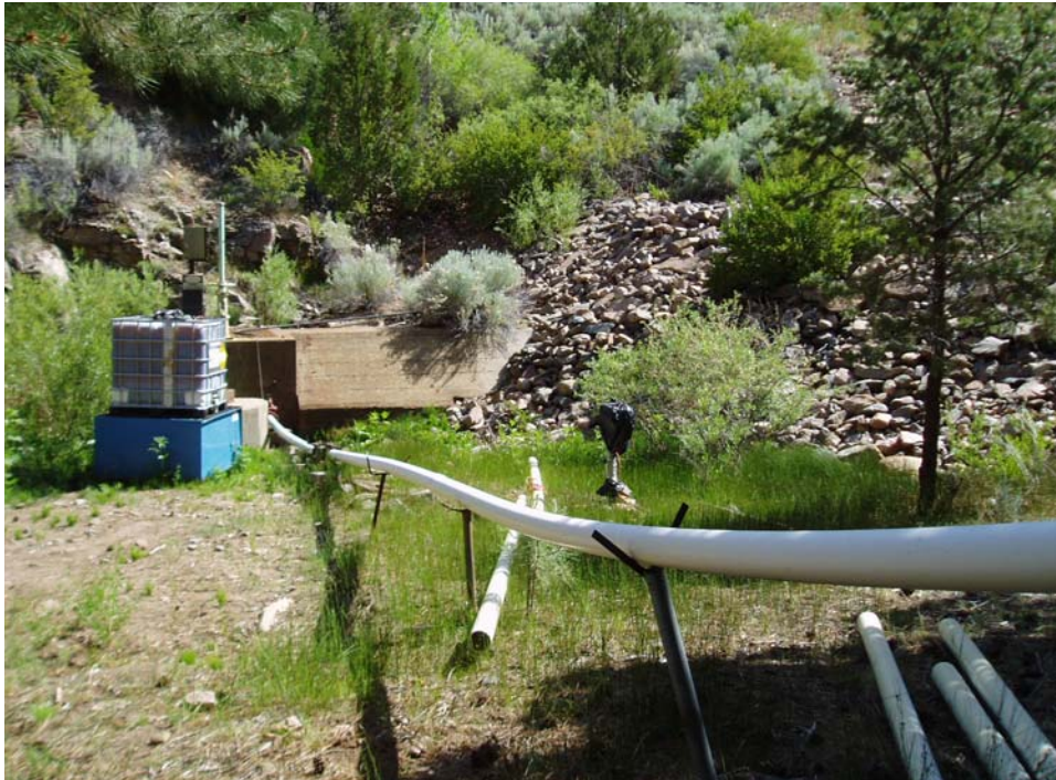
4a: Diversion structure showing toe of Nichols Dam, intake water control structure to be left in place, and pipeline running uphill to existing ditch.
