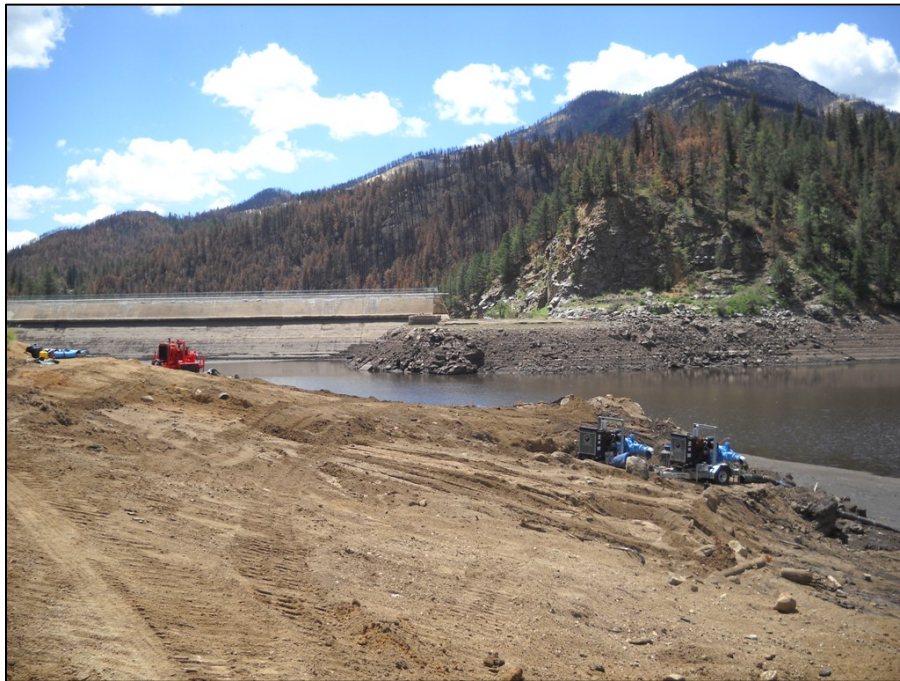
Figure 9. Photograph showing the staging area where fire debris has been cleared and lake side portable pumps have significantly lowered the lake. As lake levels are lowered, the pumps are moved lower. View approximately to S. Photograph No. 4636; 7-30-2012.
