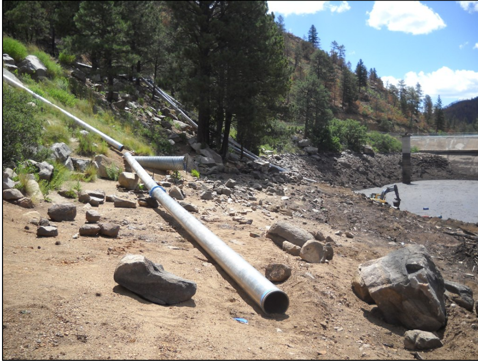
Figure 10. Photograph showing the piping from the pumps that carry water to the Bonito Lake road surface to be delivered downstream. Backhoe in the background is installing a pump closer to the lakeshore. View approximately to SE. Photograph No. 4621; 7-30-2012.
