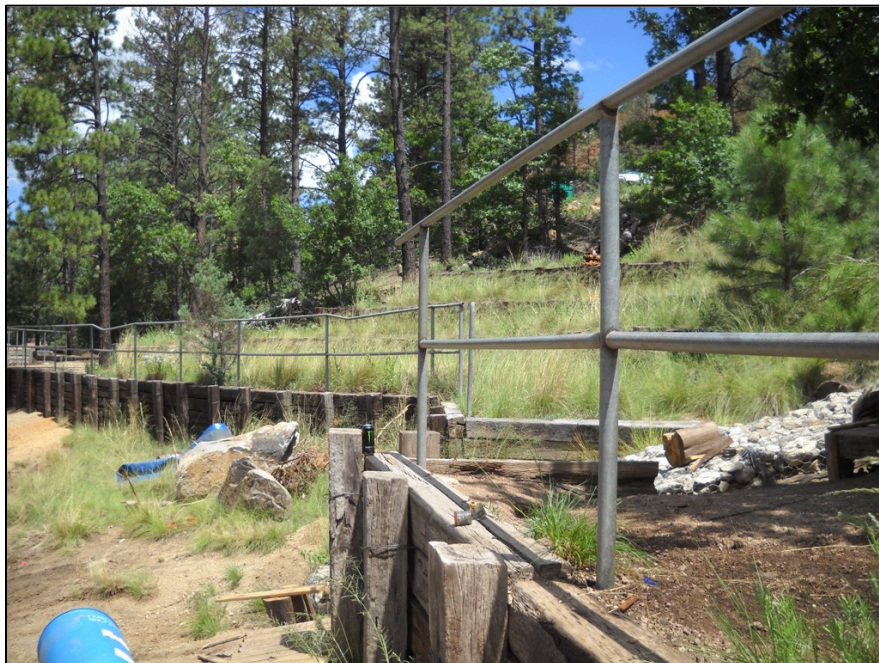
Figure 7. Photograph showing railroad-ties for hill slope stabilization, rock-filled gabion baskets for roadside rainwater drainage, and hand-railing for public access to the Bonito Lake shoreline. View approximately to N. Photograph No. 4631; 7-30-2012.
