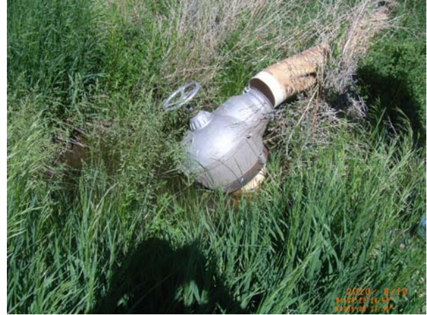
b. Leaking valve on north pipeline
