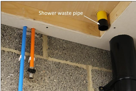
15. The shower waste pipe needs to be a \varnothing 50mm push-fit or a \varnothing 43mm O/D solvent weld pipe.
