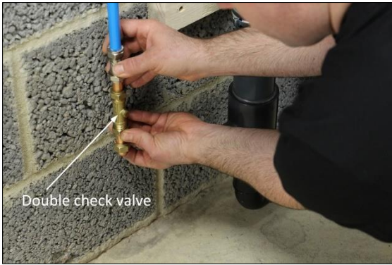
37. Connect compression fittings and copper pipe to the double check valve off the cold mains water feed.
