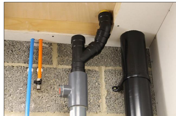
24. The combination of the T-piece and the two 45° connectors allows manipulation of the constructed coupling to achieve multiple positions to connect to the shower waste pipe.
