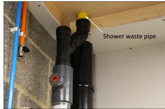
22. Connect the open end of the second 45° connector (Item 5) onto the reducer attached to the shower waste pipe.
