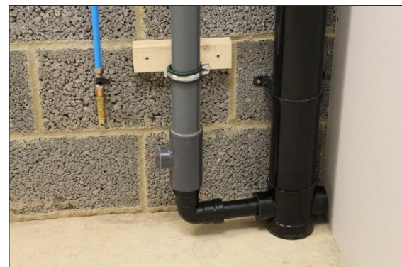
34. A straight connector is also supplied (Item 6) for installations where the soil stack connection is below the floor level.
