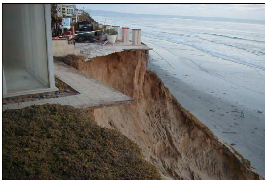
Figure 1.4-2 Example of damage to structure and land loss at bluff top edge
