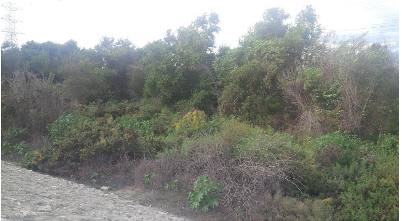
Figure 3. The accumulated sediment and vegetation that is impinging the flows from San Jose Creek.
