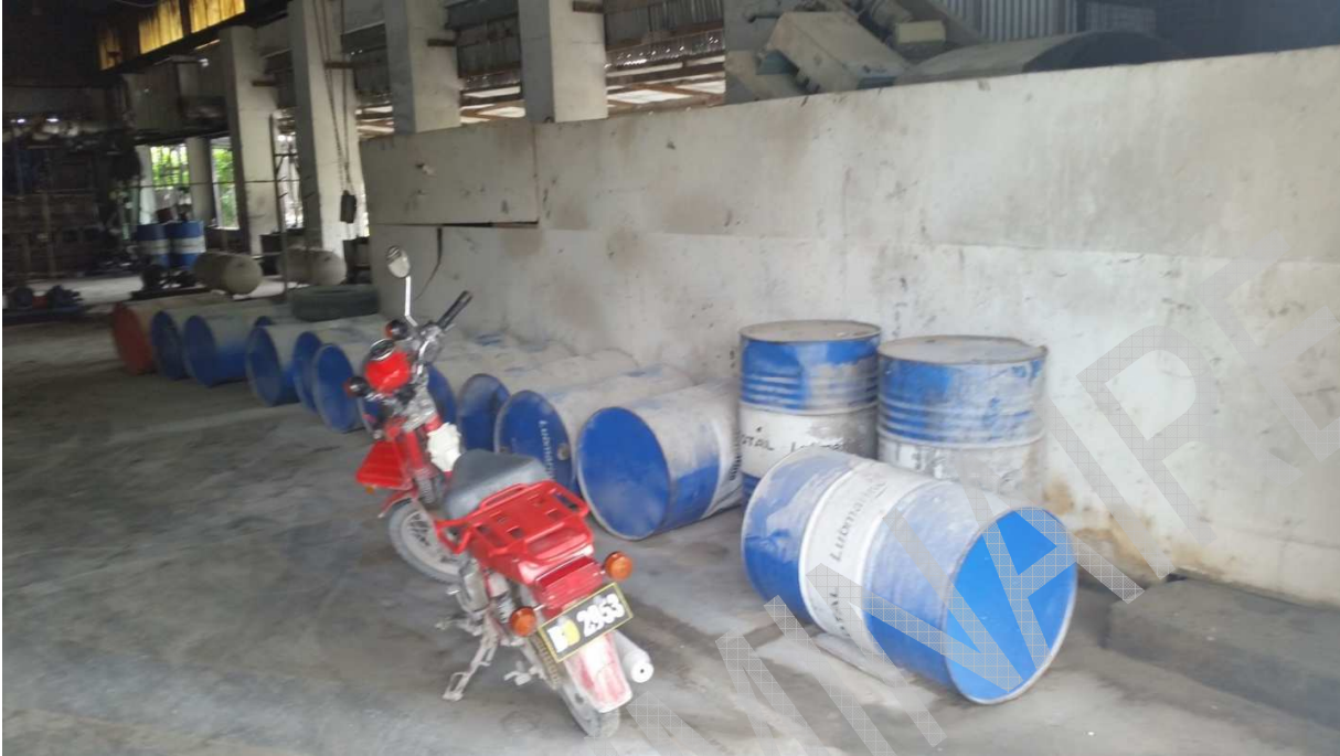
Figure 3: PUB Betio Power Station (Storage of Lube oil)
