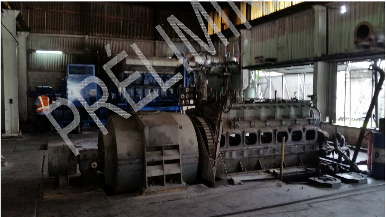
Figure 2: PUB Betio Power Station (generator)
