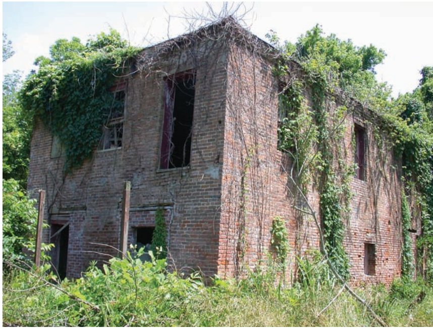
Figure 5—Abandoned building in Jefferson County, MS, recently discovered as a roost site for > 150 Rafinesque’s big-eared bats. (Photo by Chester Martin)
