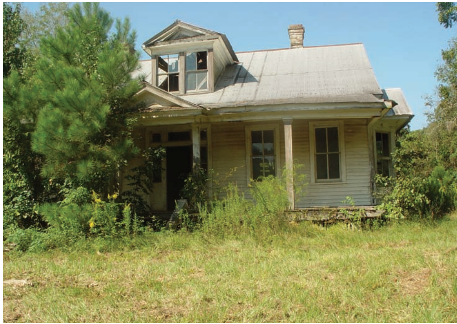
Figure 3—Abandoned house on St. Catherine Creek National Wildlife Refuge that historically served as a maternity roost for 40 to 60 Rafinesque's big-eared bats. (Photo by Alison McCartney)
