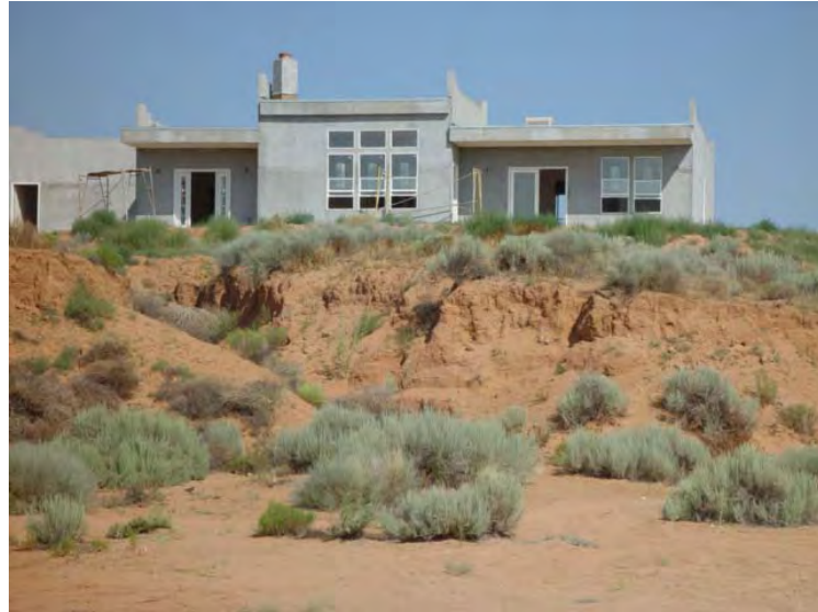
Photo 14 - House possibly in lateral erosion limit
