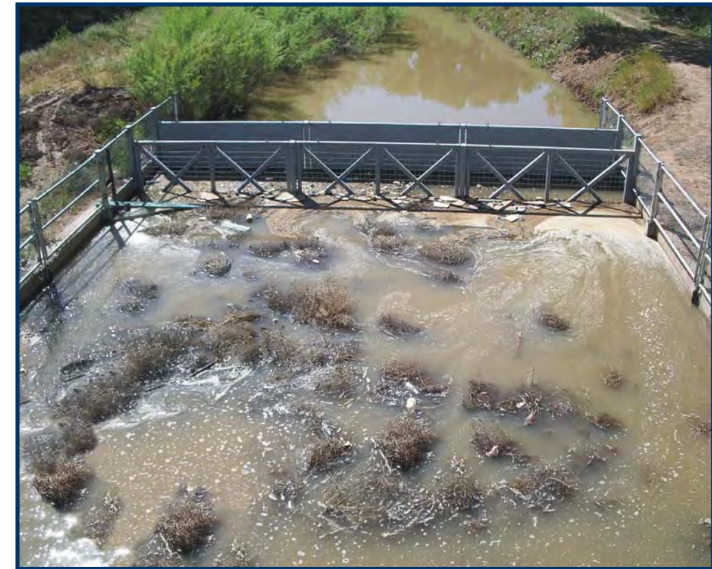
Photo 13 - Gross Pollutant and Floatable Control Facility
