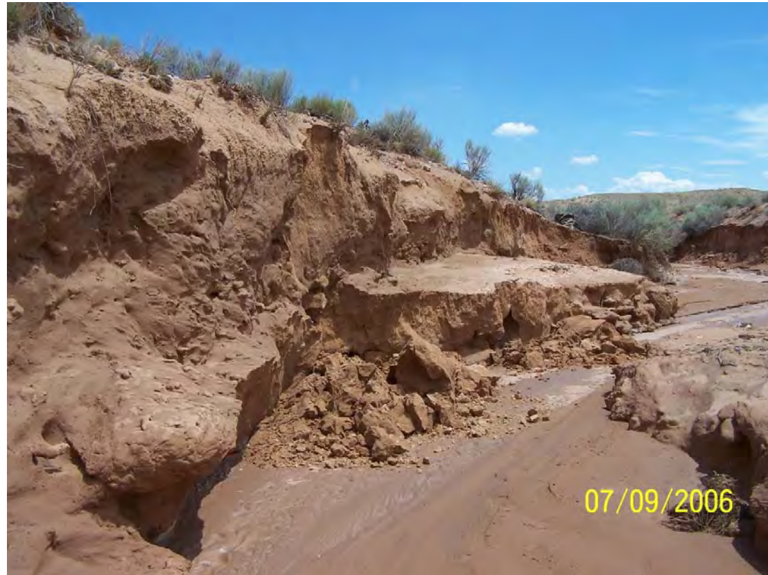
Photo 9 - Tributary BAK Following July 8, 2006 Storm
