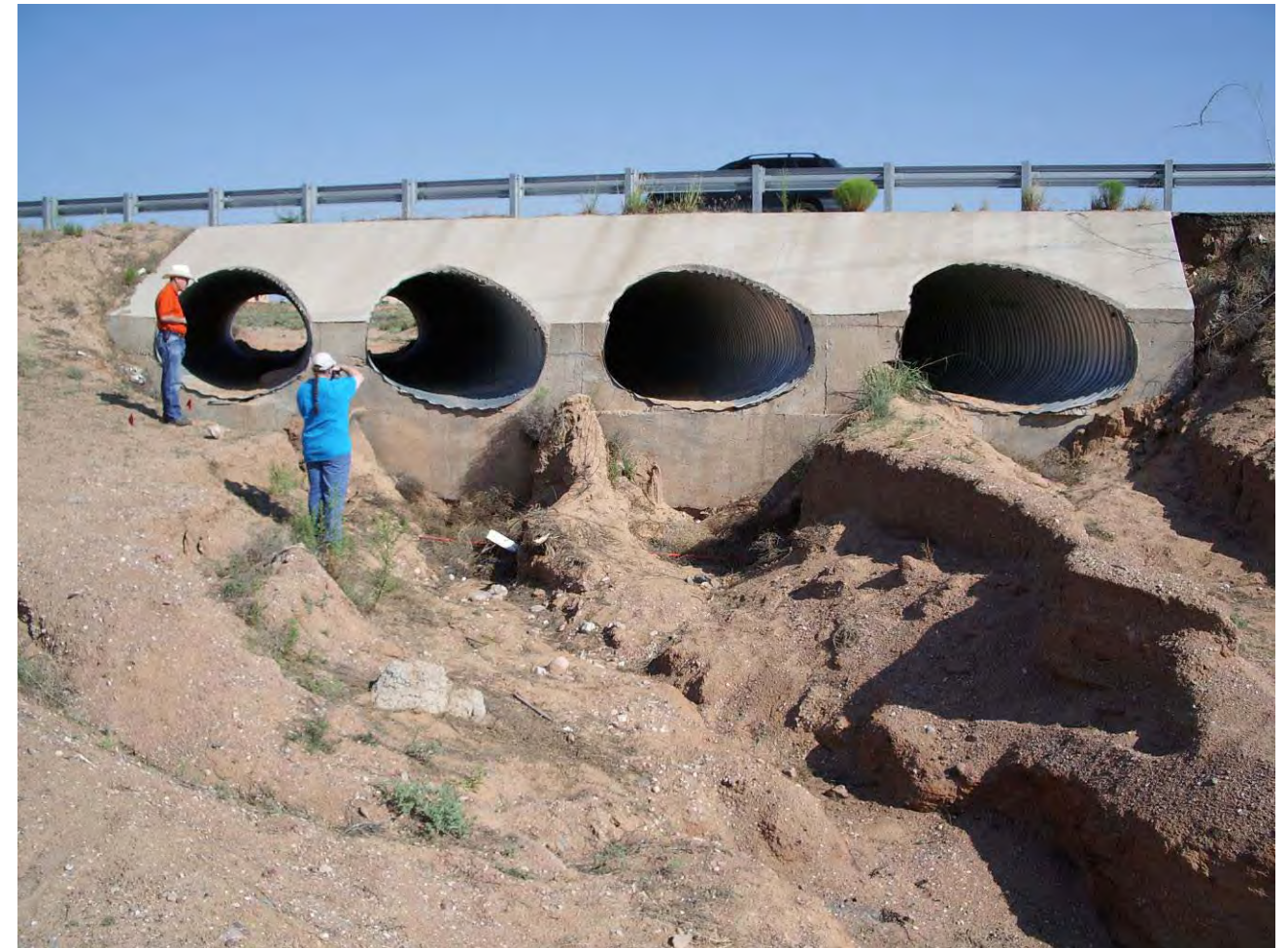
Photo 3 - David Stoliker and Karen Jacobsen inspect erosion Main Branch outfall at Idalia Rd.
