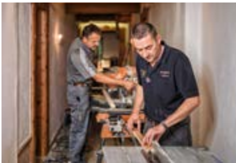
Hauseigene Experten. Der Stanglwirt-Bautrup in Aktion. In-house experts. The Stanglwirt construction crew in action.
