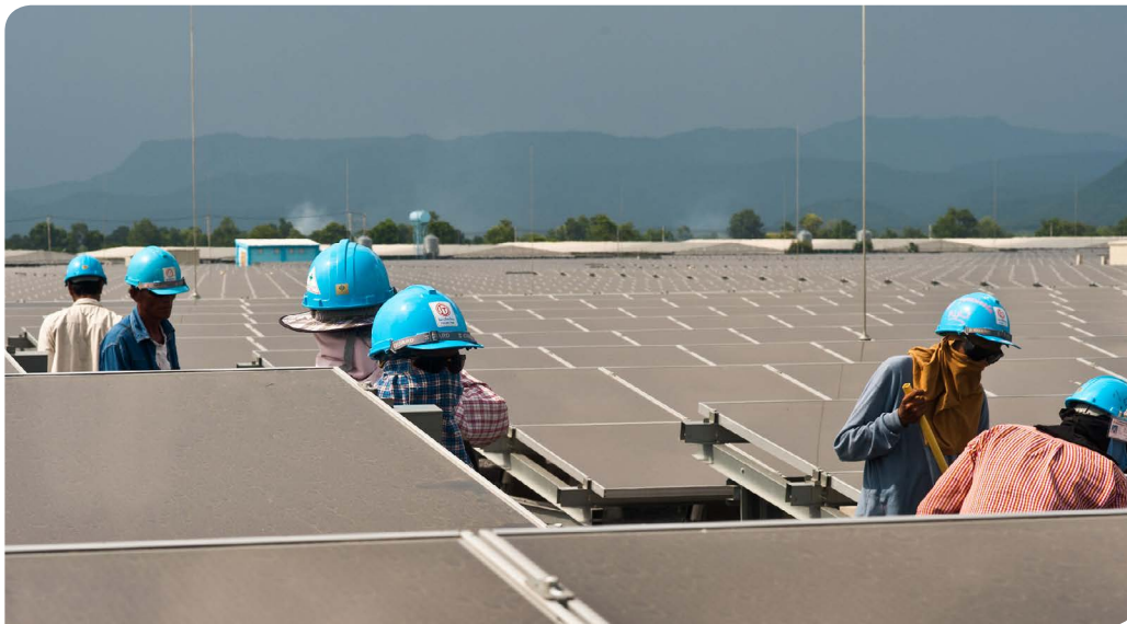
Above: Solar power project in Thailand, courtesy of the Asian Development Bank
