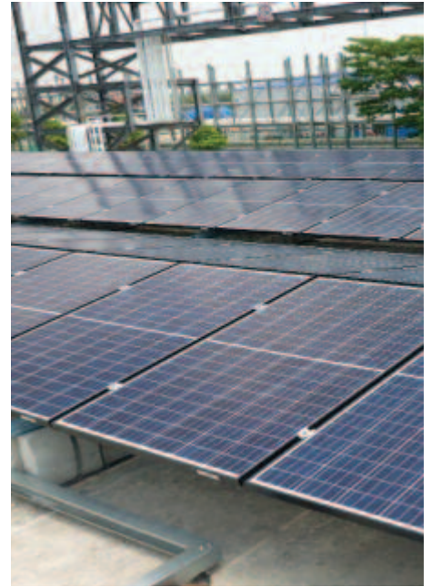
The solar panels installed on the roof of Stolthaven Singapore's administrative building.
