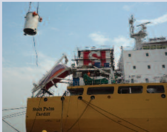
Scrubbers being lifted on board and installed on Stolt Palm (top) and Stolt Maple (bottom).
