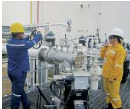
Kong Jia Yin, right, supervising pigging operations in the tank farm area.
