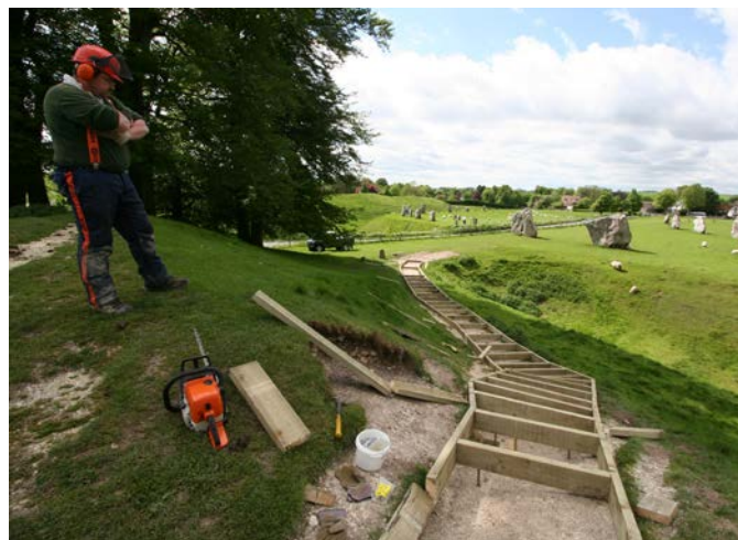
'Drapes' laid over the monument to protect it from erosion by visitor footfall
