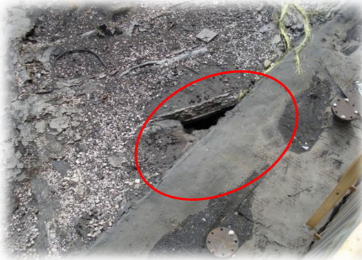
ESP Outlet duct
