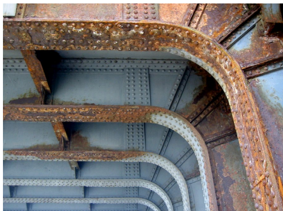
Photo 1 : Corrosion © JP Persy
