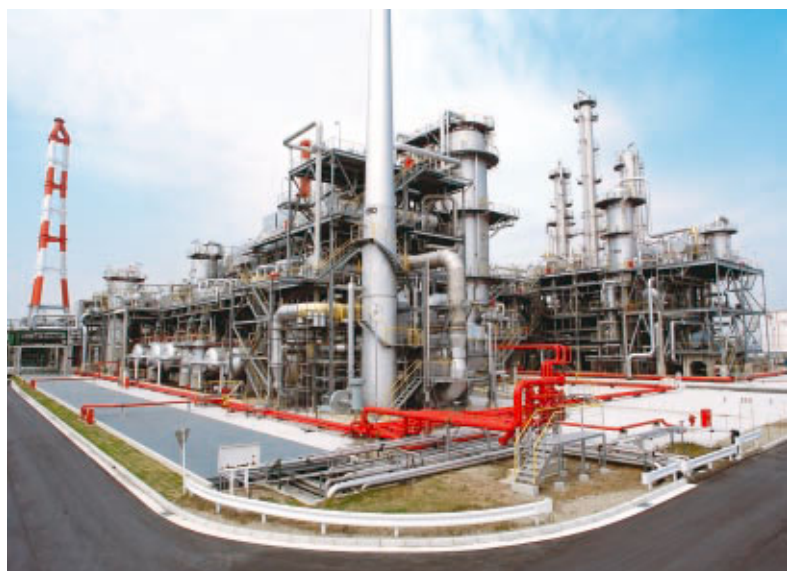
The new plant uses a novel production process to manufacture PO with no co-product.
