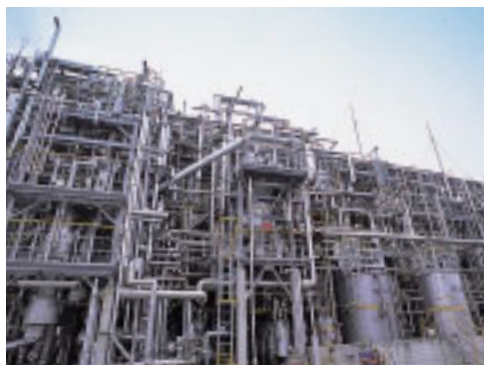
Pilot facility for caprolactam production
