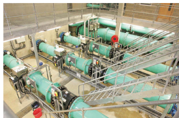
▲ Sutton & East Surrey Water's Elmer treatment works in the U.K.
