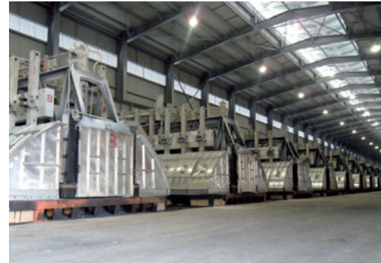
▶ Electric furnaces for smelting aluminum ingots at Press Metal Berhad in Malaysia
