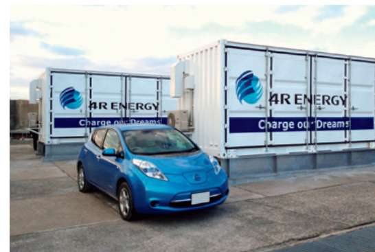
Large-scale power storage system utilizing used EV batteries
