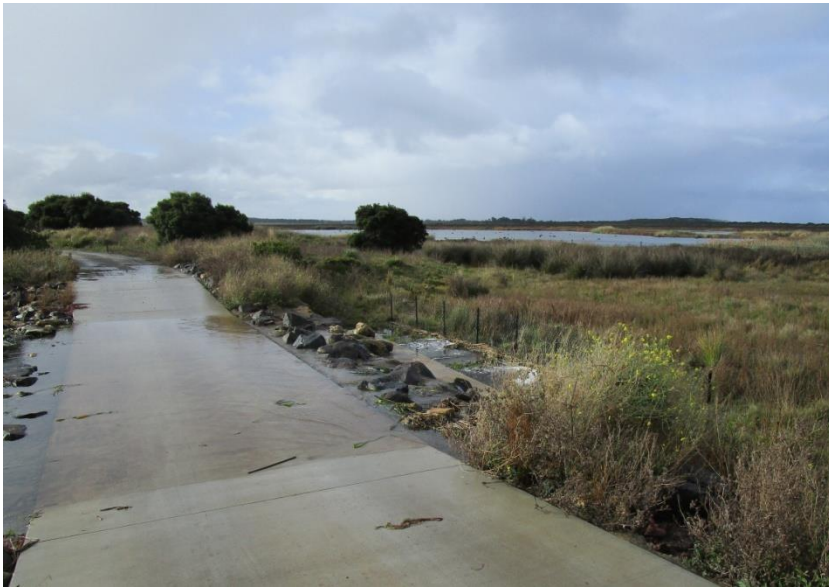
Stormwater flowing over the spillway between the stormwater treatment pond system and the Karaaf.
