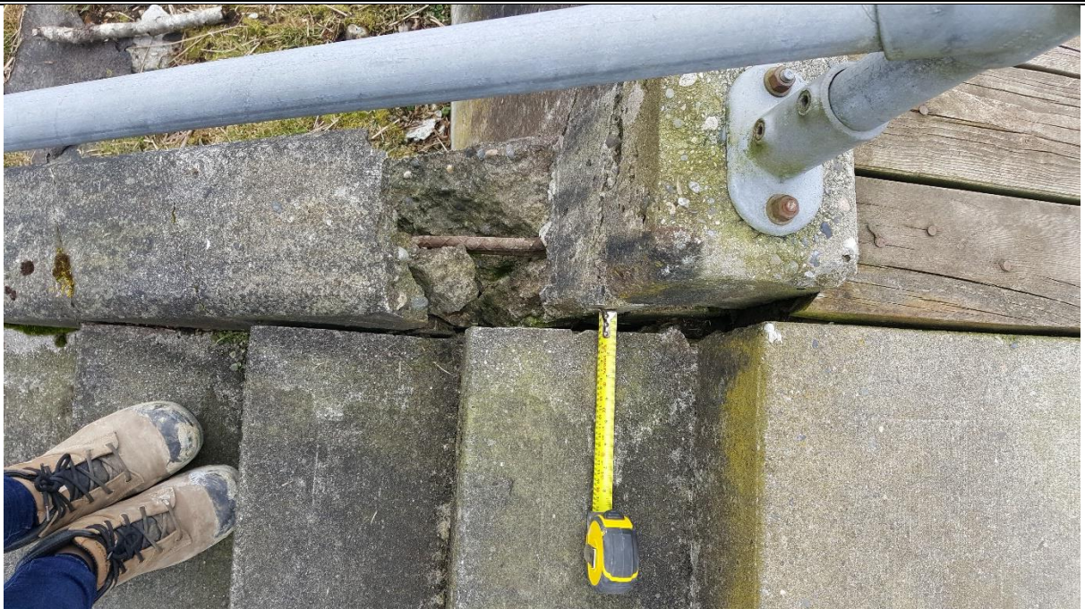
Photo 3 – Gap between the stairs and retaining wall for Erikson Pump Station.
