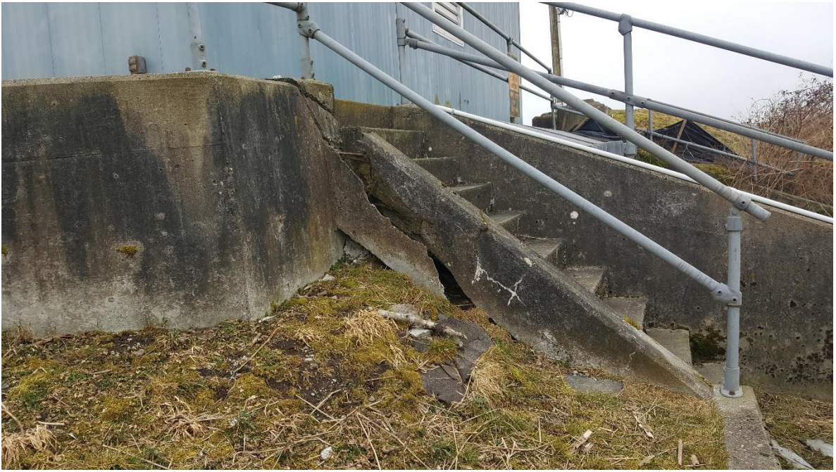
Photo 1 – Failure in north stair stringer for Erikson Pump Station.
