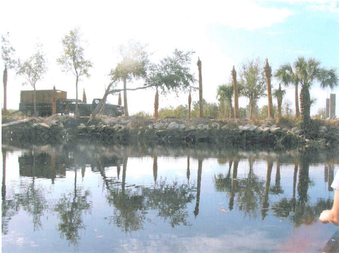
Figure 25: An example of new construction with rubble used to armor the shoreline at RK15.
