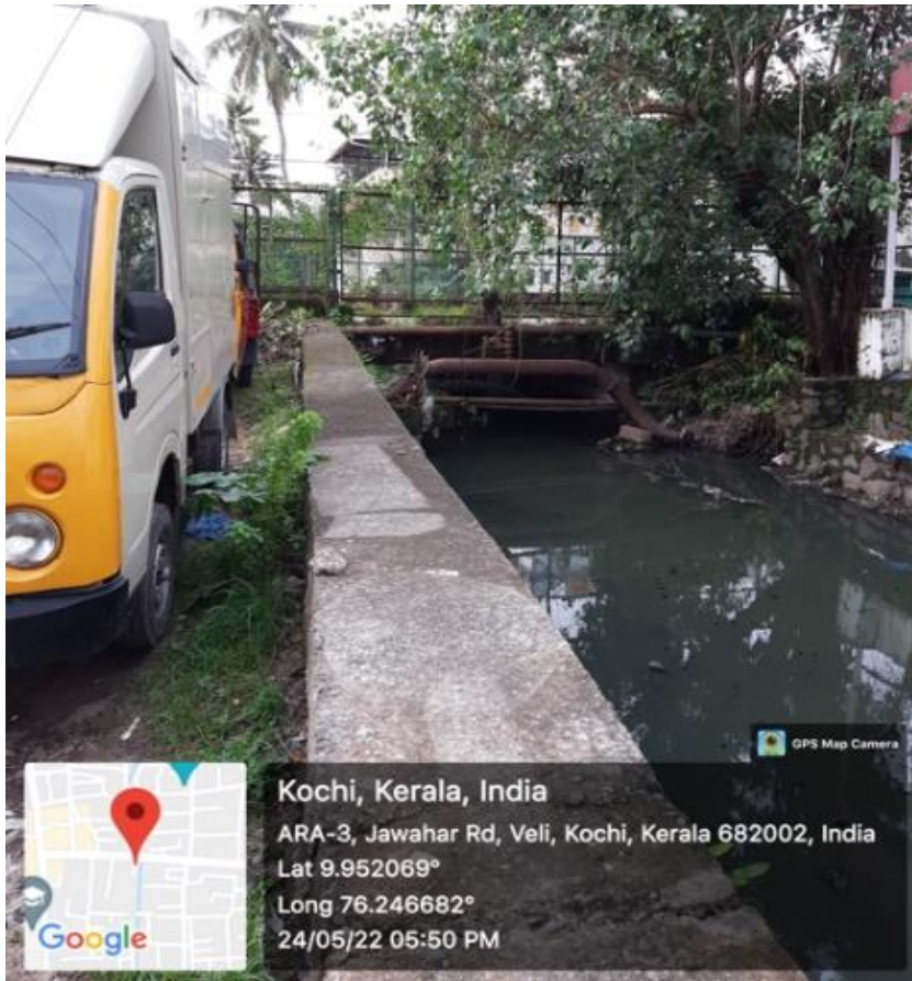
KWA Water pipeline aligned across the canal. At high flood levels in the canal the water pipeline can come in direct contact with the polluted canal water (Photo Credit: bechtel.org)
