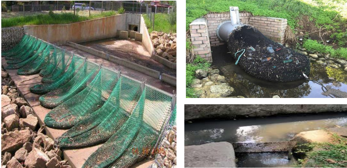
Figure 17: Trash Screens (Photo Credit: bechtel.org)
