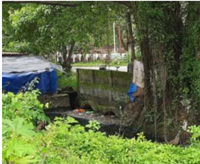
Figure 4-9: Blockage due to accumulation of solid waste
