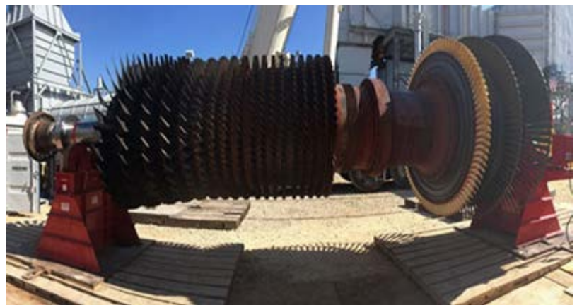
Figure 1: GE 7FA rotor during maintenance.
