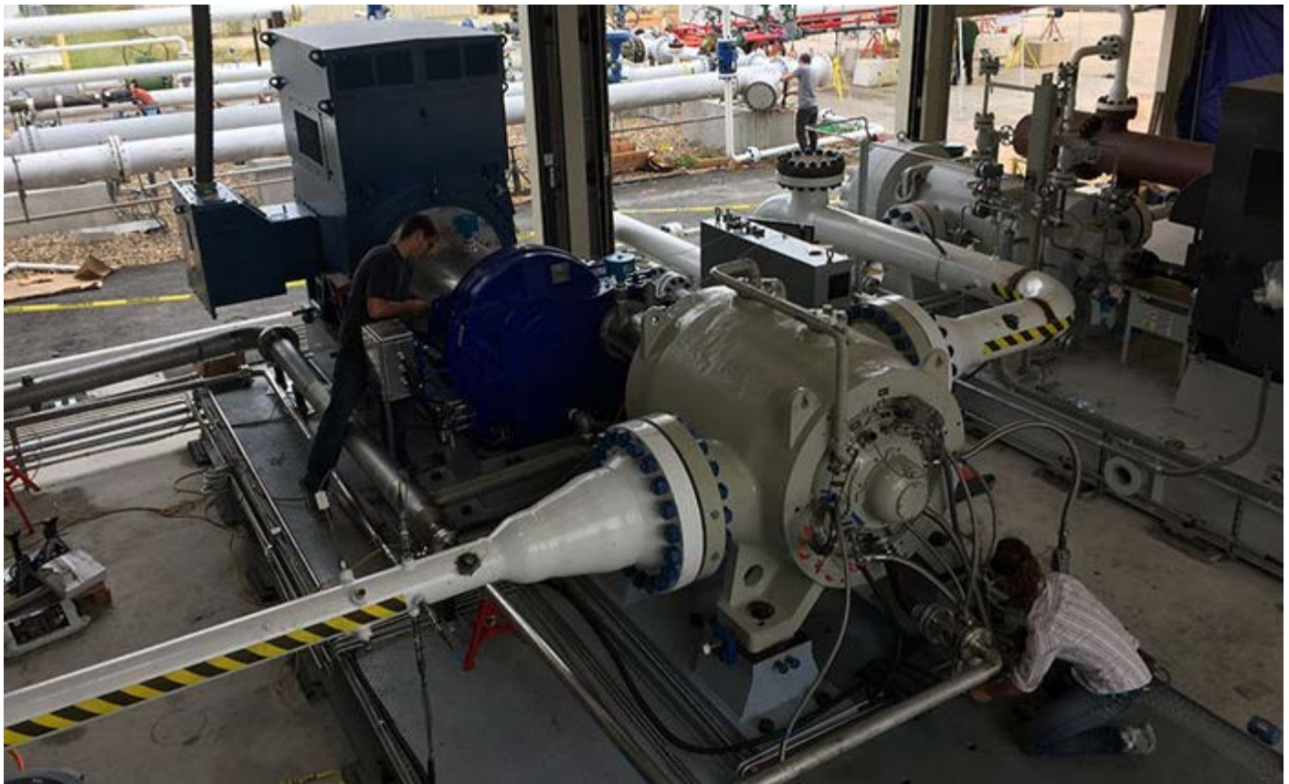
Figure 1: C33 compressor during commissioning.
