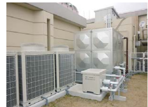
The energy efficient hot water heater EcoCute is installed in the caregiving facility "St. Joseph's Garden"
