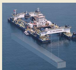
World's first working vessel for constructing RC immersed tunnel element on the sea and immersing them
