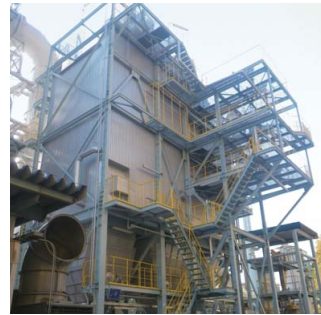
Waste heat boiler
