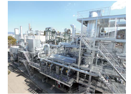
Sewage sludge-fueled power plant
