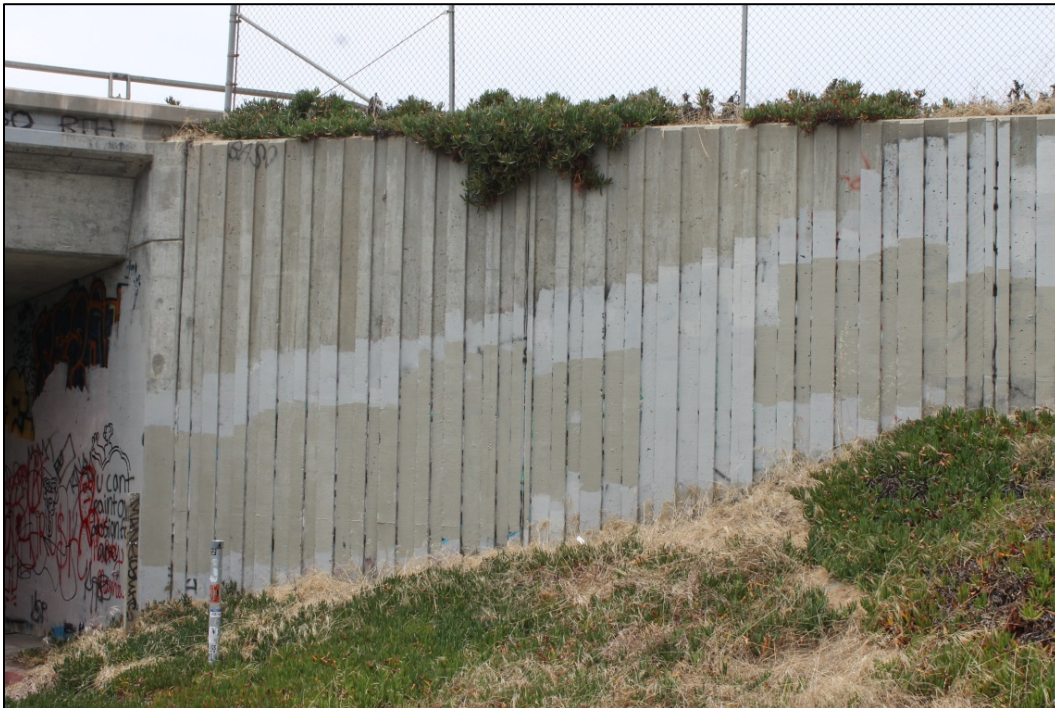
Photograph 10. Detail of bridge with graffitied walls and unmaintained iceplant on land adjacent to Divarty Street. Alignment would occur adjacent to this area.
